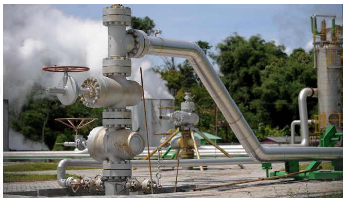
Figure 5. Pipes used during the transport of water in a geothermal power plant. ‡
