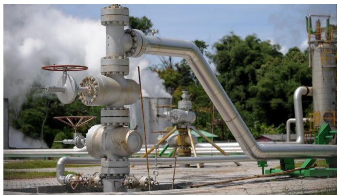
Figure 5. Pipes used during the transport of water in a geothermal power plant. ‡
